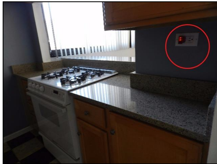
10. No GFCI/GFI (Ground Fault Circuit...
