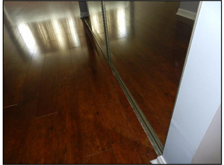
30. Loose or poor fit
