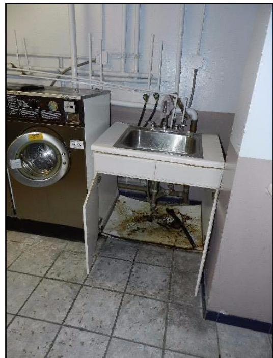
21. Leak @ Laundry Sink
