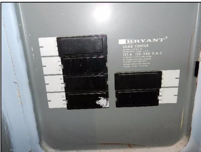
2. No fuses or breakers for subpanel (pony...
