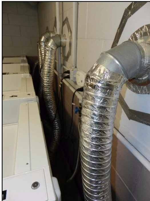
35. Dryer vent material not smooth wall
