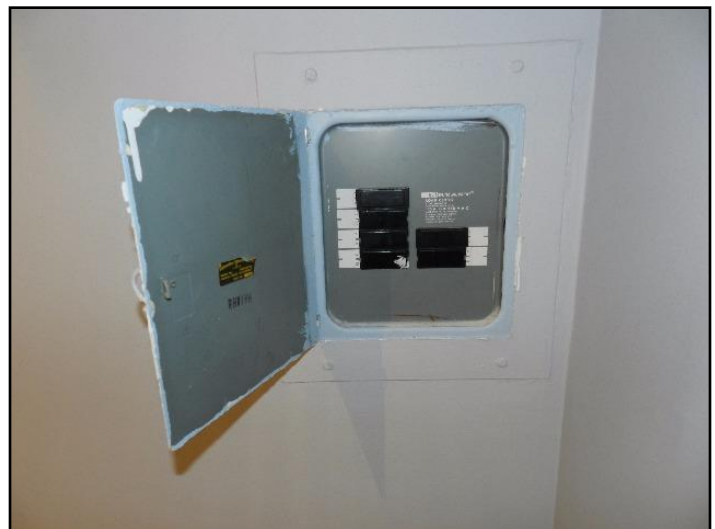
3. No fuses or breakers for subpanel (pony...
