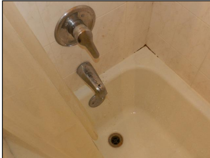
22. Caulking loose, missing or deteriorated
