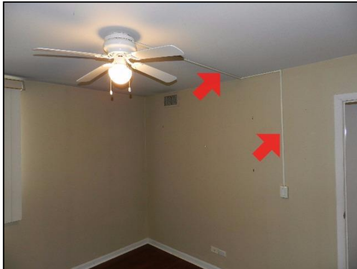
4. Exposed on walls or ceilings
