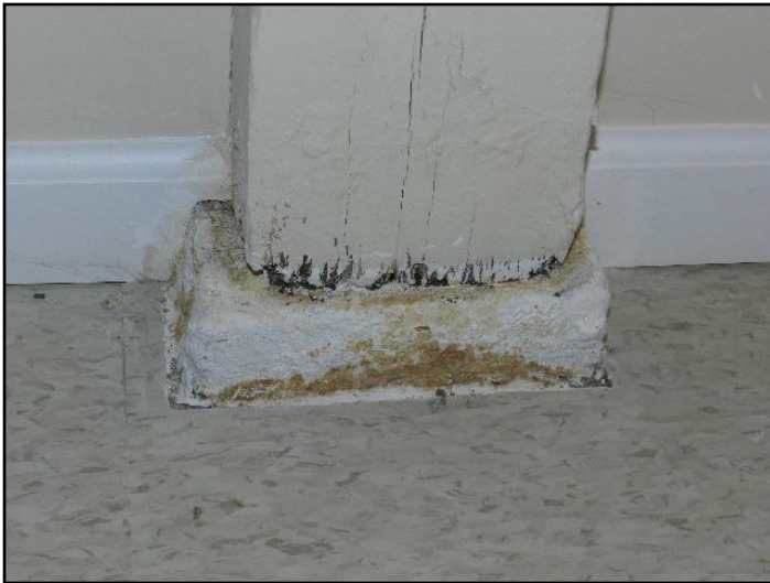
124. Wall cracks with water stains
