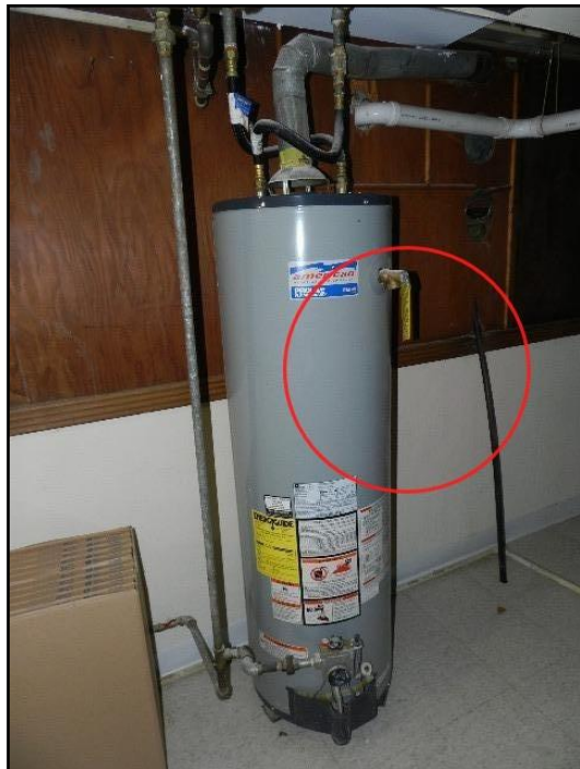
76. Discharge tube missing
