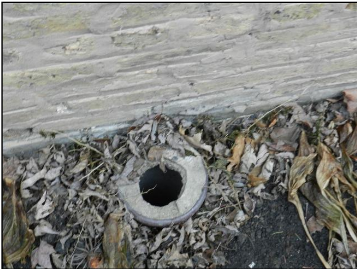
83. Uncapped drain to sewer, possible backup
