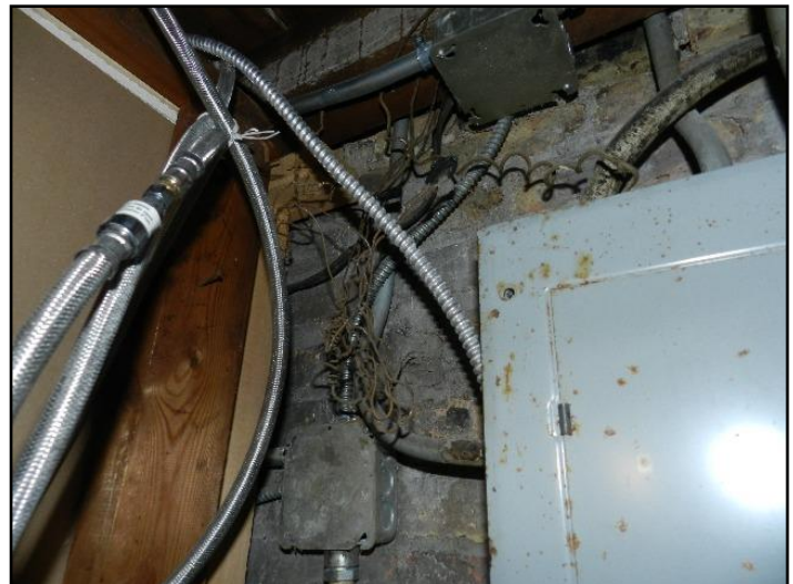
44. Wrong type, tape wiring, Romex
