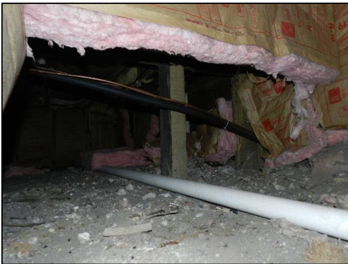
64. Exposed combustible insulation
