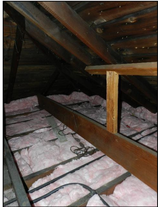
61. Exposed combustible insulation
