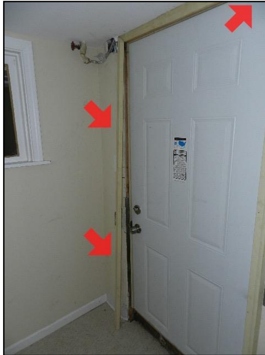
107. Poorly fit, loose
