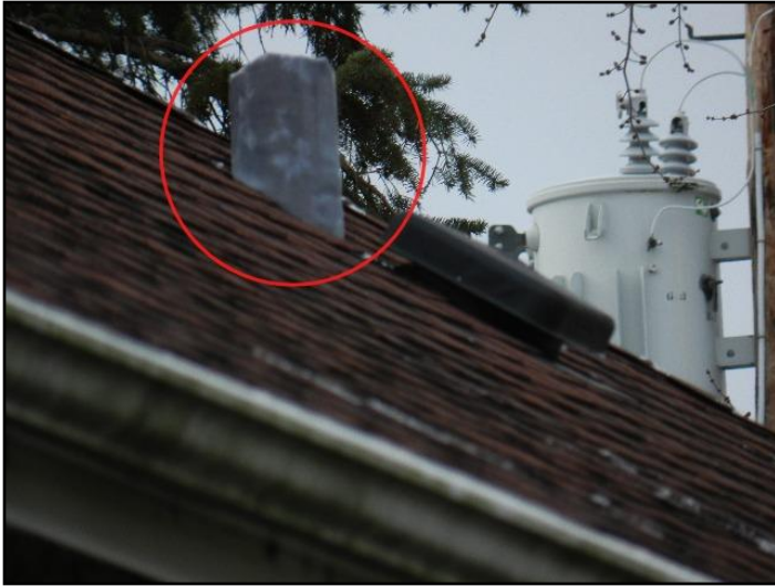
4. Missing flashing and cap
