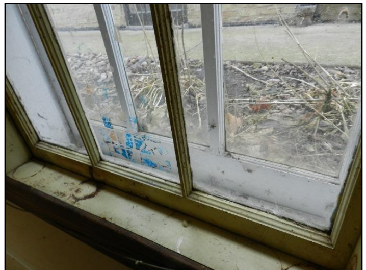
19. Air, water leaks
