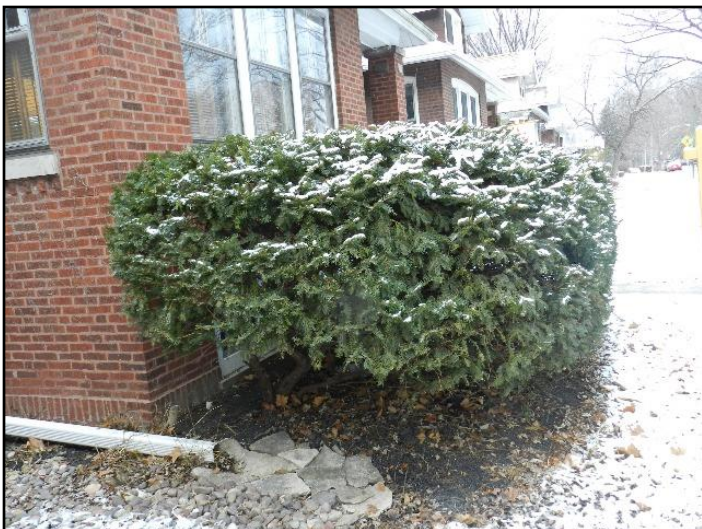
25. Overgrown shrubs too close to building
