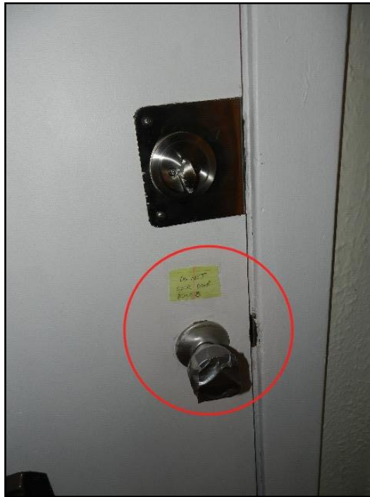
106. Lock not effective on exterior door
