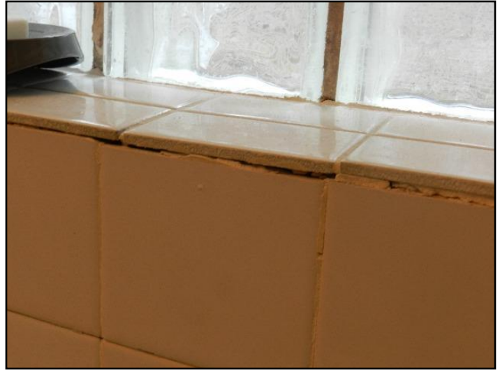
89. Grout loose, missing or deteriorated
