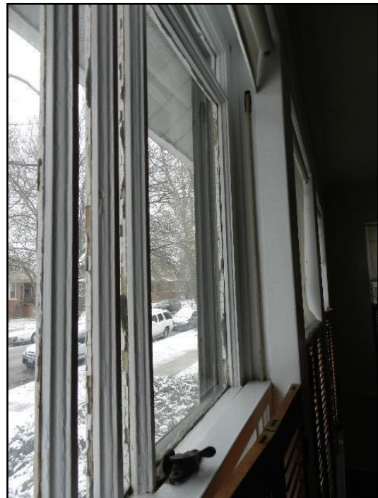
15. Air leaks, does not lock
