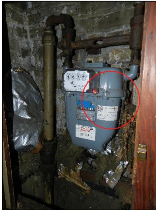
74. Gas odor around meter
