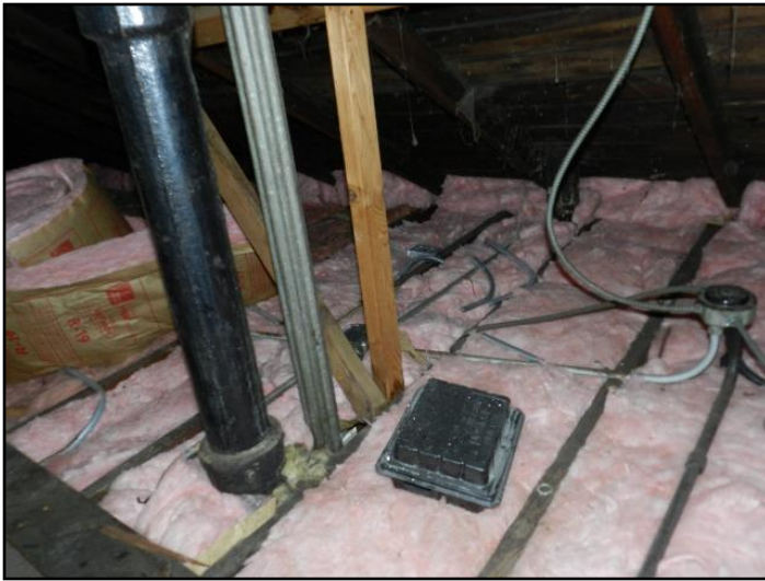
60. Pest droppings,exposed combustible insulation
