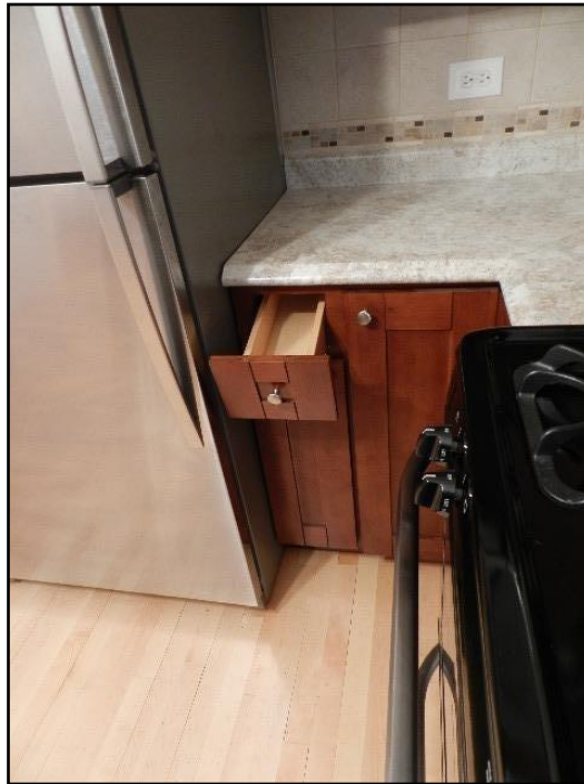
108. Doors or drawers missing or loose
