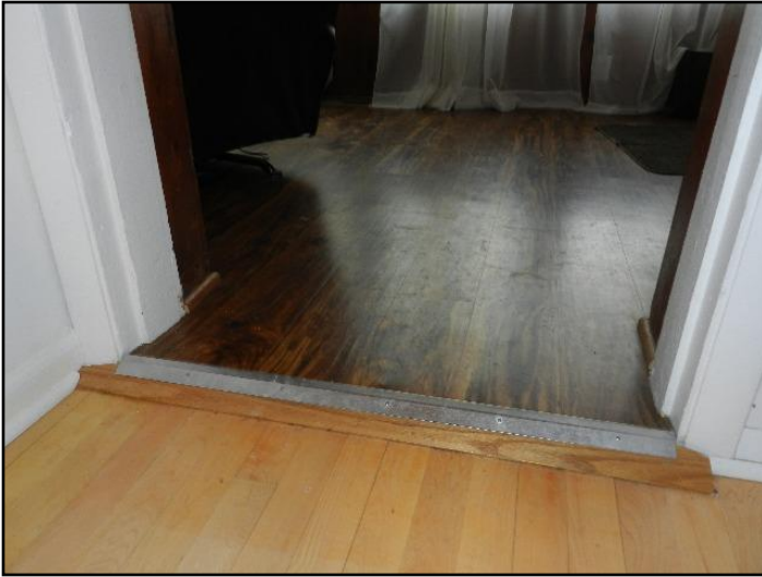
95. Trip hazard, uneven floor levels
