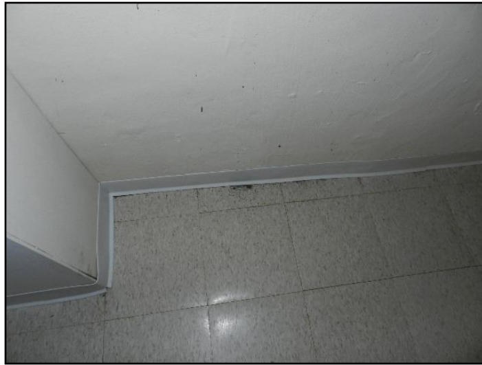
118. Loose floor tiles
