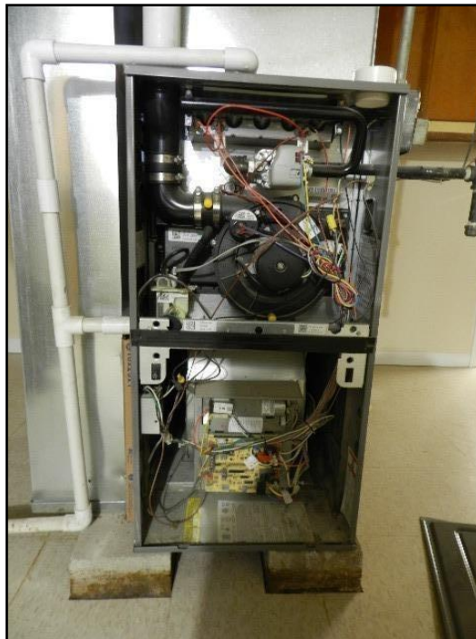
49. Inadequate combustion air
