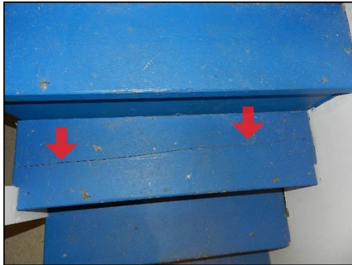
114. Worn or damaged
