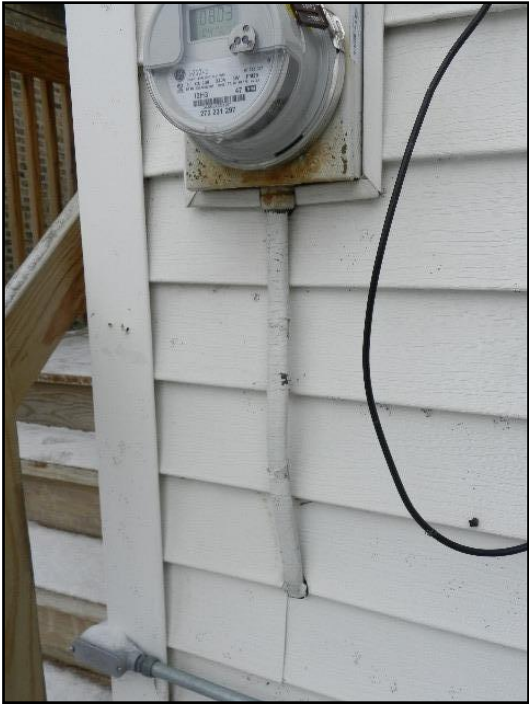
41. Conduit or cable not weather-tight
