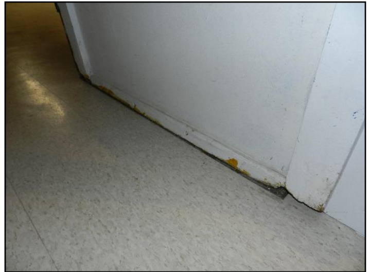
125. Wall cracks with water stains
