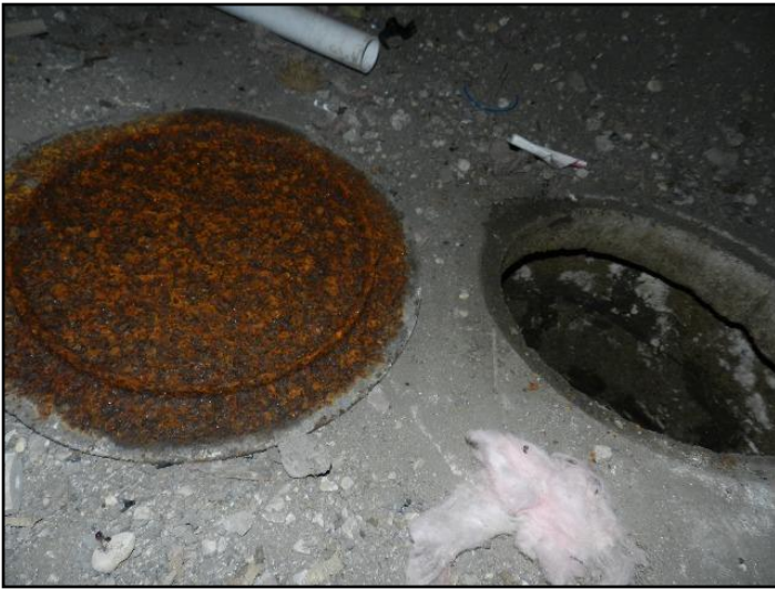
85. Rusted cover at catch basin
