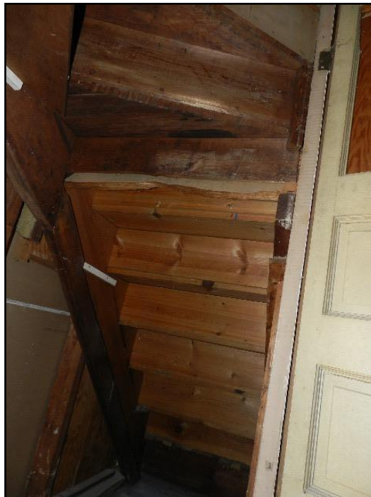
109. Drywall missing or incomplete on underside...
