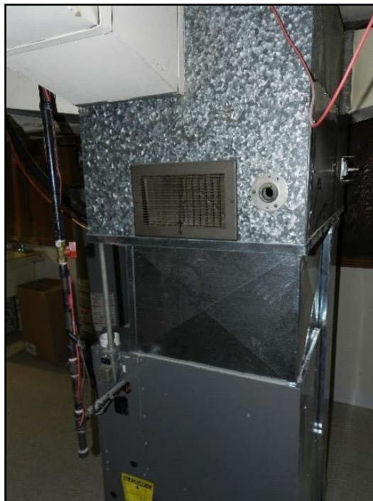
58. Opening and grille in supply duct by furnace
