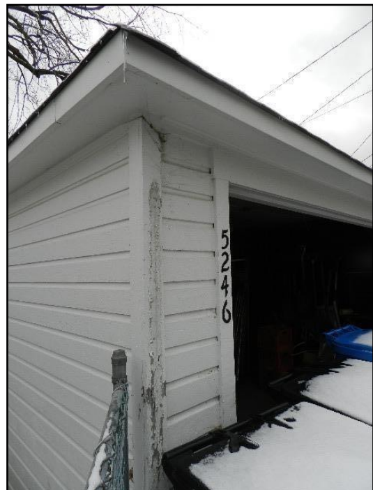
30. Gate does not open, paint needed at garage
