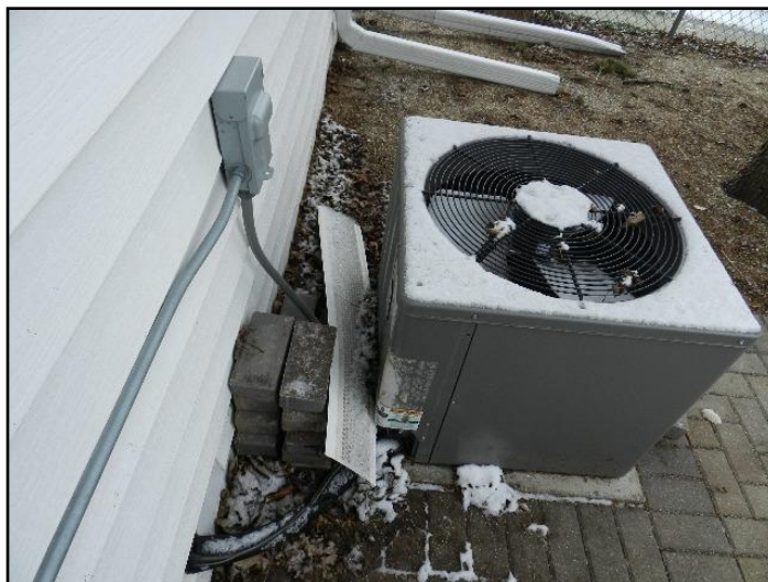
54. Condenser not covered/protected from snow/ice
