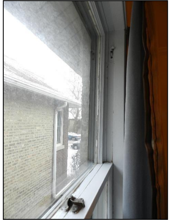
21. Air leaks, does not lock
