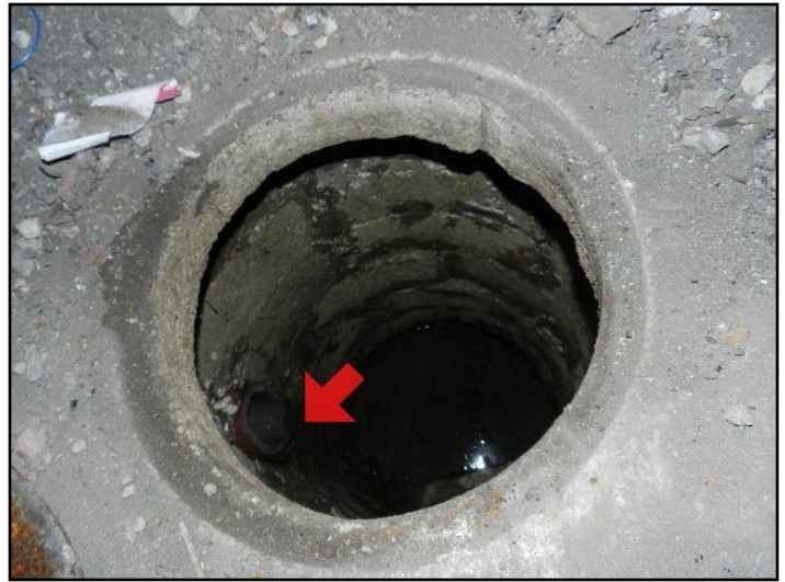
86. Backup, no check valve
