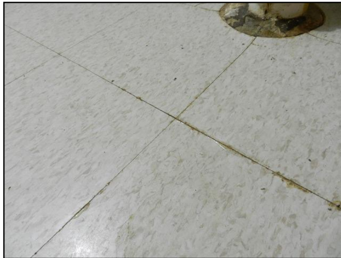
132. Possible vinyl-asbestos floor tiles
