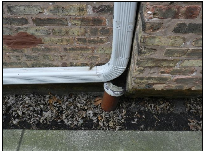
84. Uncapped drain to sewer, possible backup
