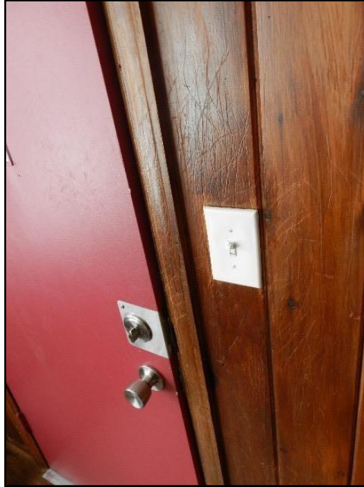
94. Damaged, dog scratches at wall
