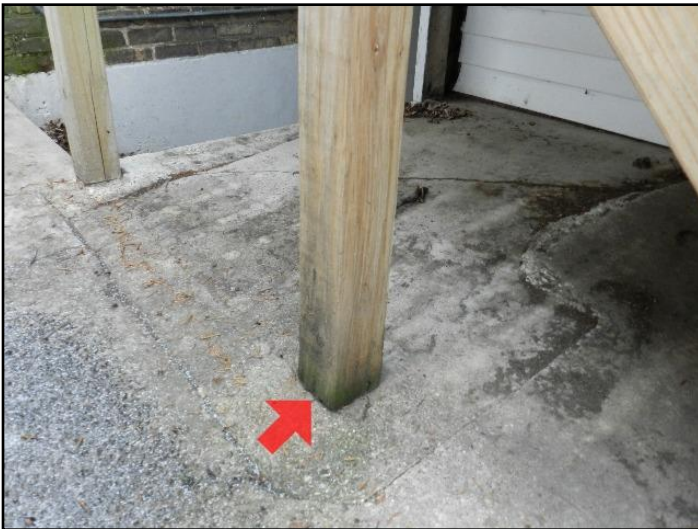
22. Rot, no footing
