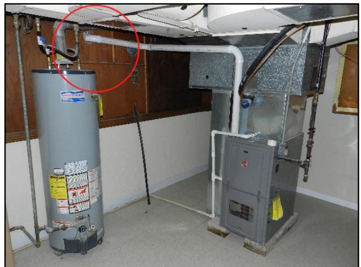
51. Poor vent location, arrangement
