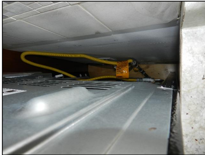
130. Anti-tip device missing
