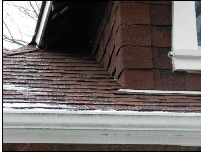
3. Side flashings not set into shingles properly
