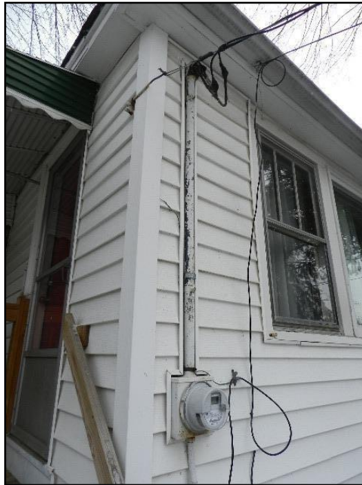
40. Old, inadequate electrical service size
