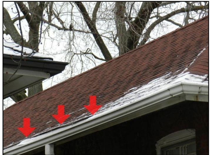
7. Loose or damaged
