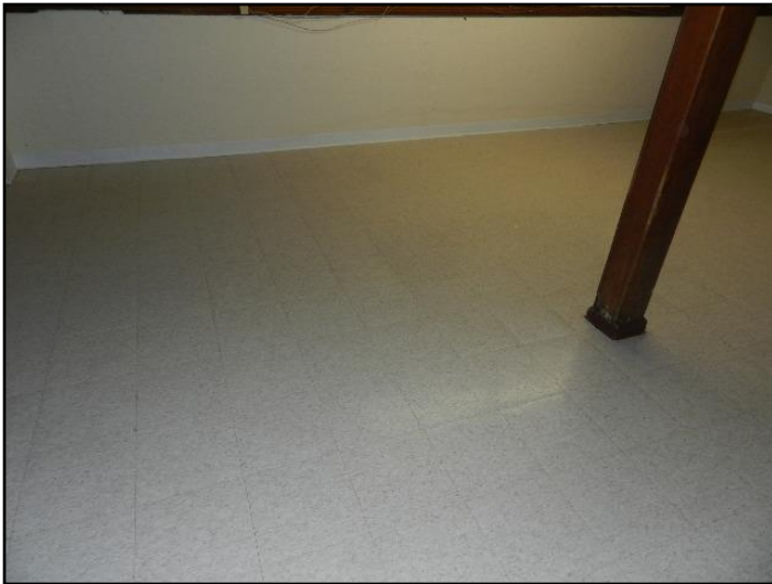
116. Loose floor tiles
