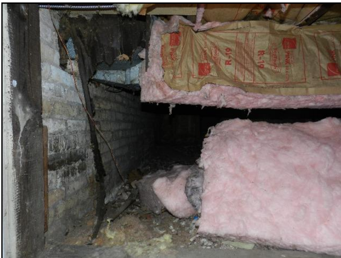
68. Wet, exposed combustible insulation
