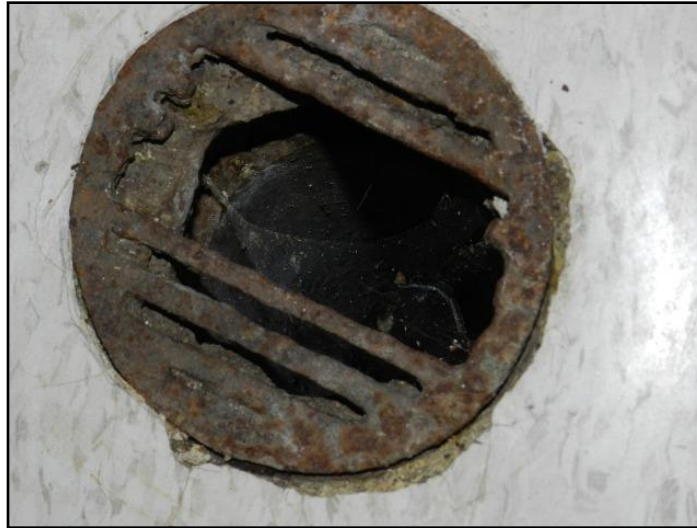
82. Grate missing, rusted or obstructed
