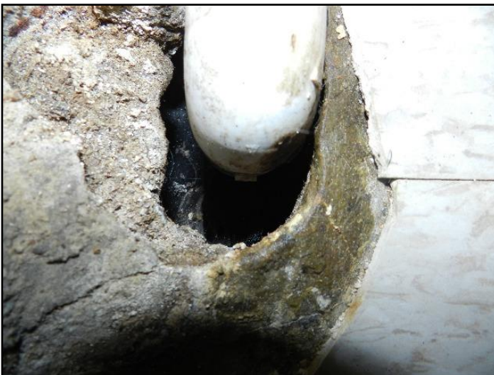
80. Missing - incorrect condensate draining
