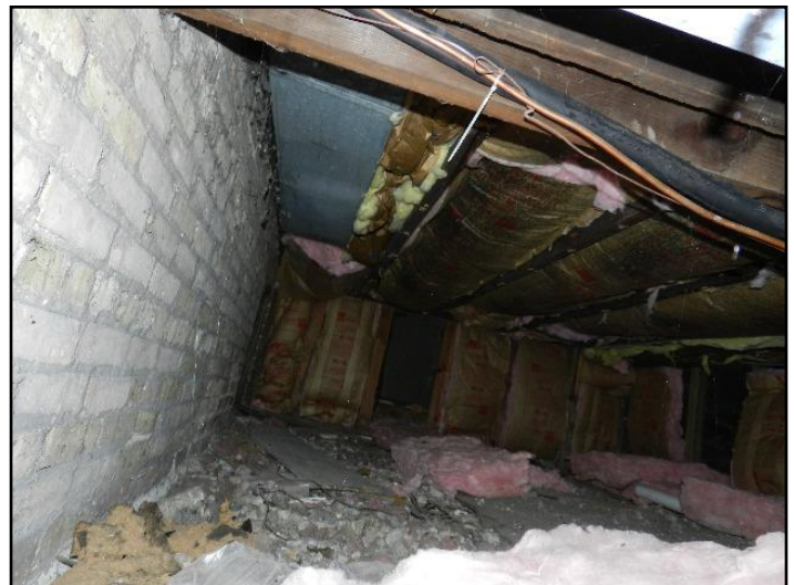
69. Exposed combustible insulation
