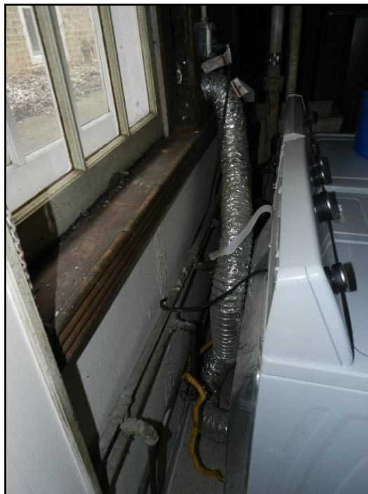
131. Dryer vent material not smooth wall
