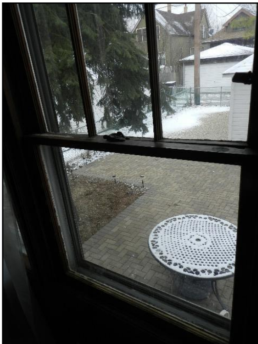
18. Air leaks, does not lock
