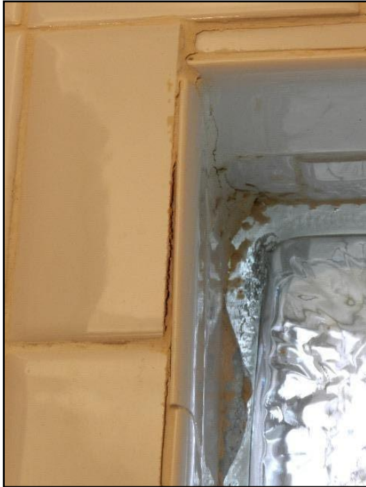
88. Grout loose, missing or deteriorated
