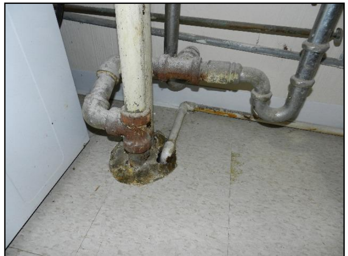
81. Missing floor drain at furnace & water heater
