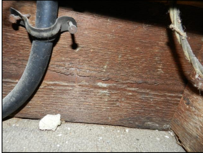
59. Return chase or plenum contain pipes, wires...
