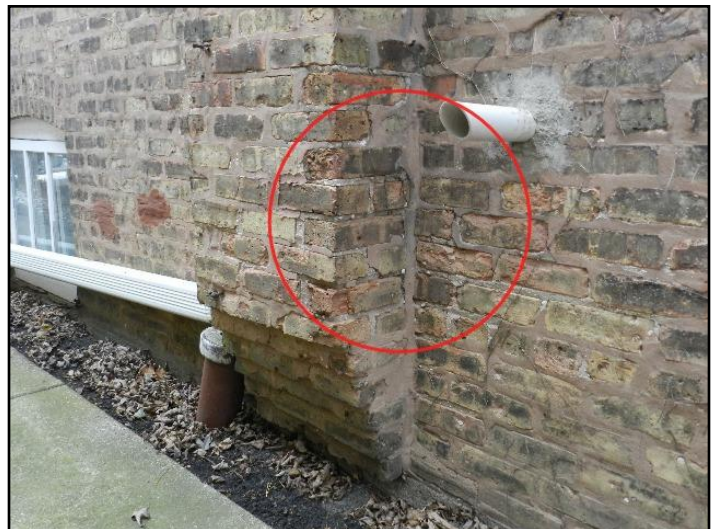
12. Sulfuric acid fumes damaging masonry
