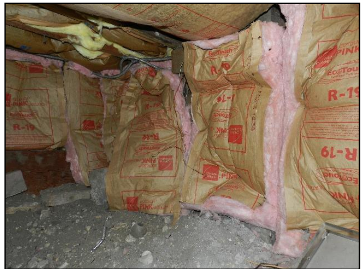
65. Wet, exposed combustible insulation
