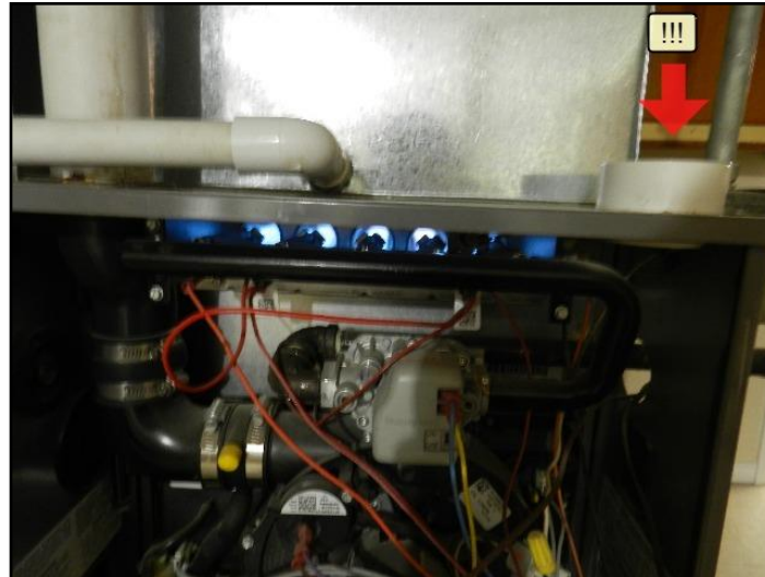
52. Poor combustion air intake location
