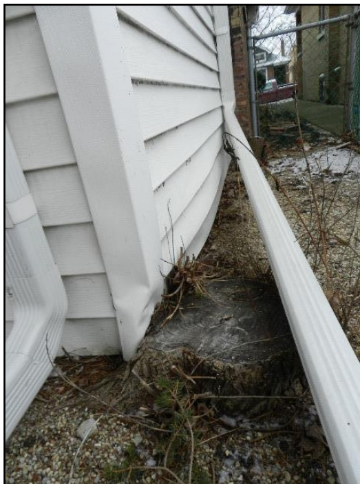
26. Trees trunk too close to building
