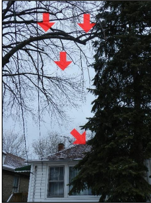
1. Tree branches above roof structure
