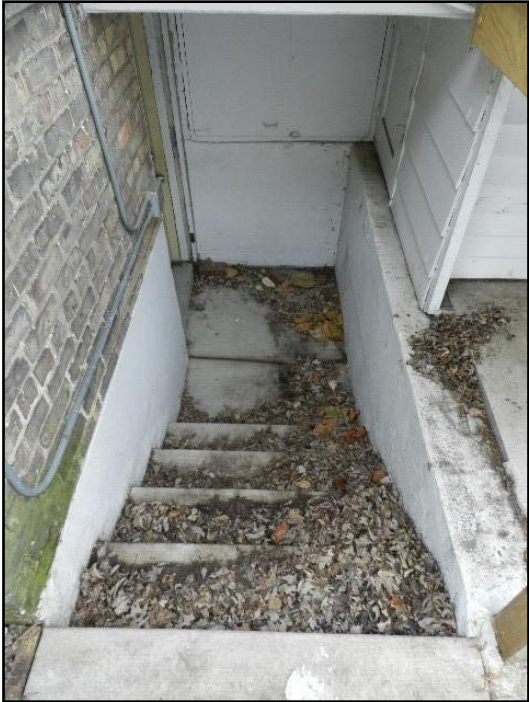
24. Guard and handrail problems
