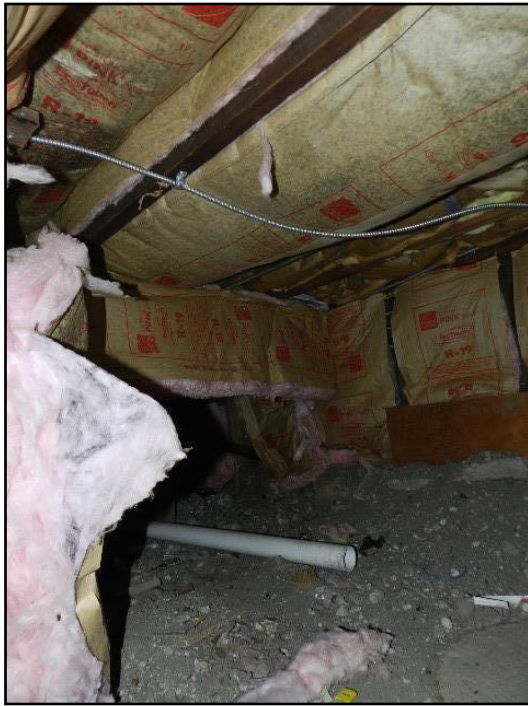
66. Exposed combustible insulation
