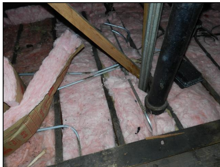
62. Pest droppings,exposed combustible insulation
