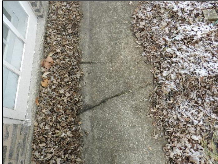
28. Cracked or damaged surfaces
