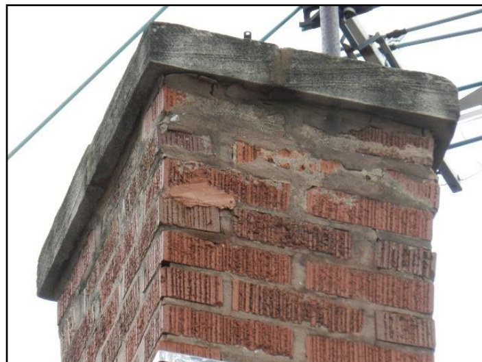
53. Loose, missing or deteriorated mortar
