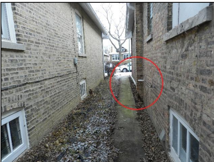
50. Poor vent location, arrangement
