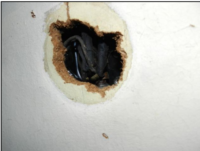
43. Wrong type, old tape wiring
