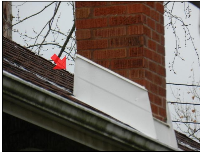
2. Cricket missing, loose, damaged
