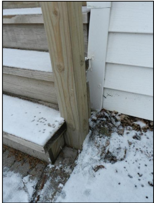
23. No footing, wood/soil contact
