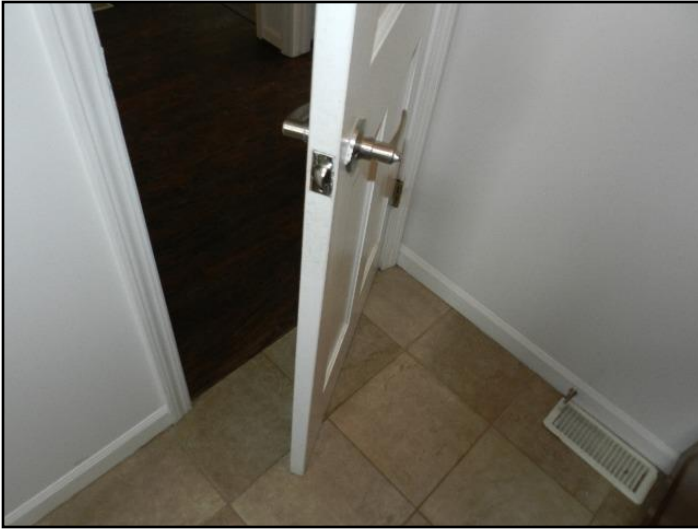
103. Privacy lock broken
