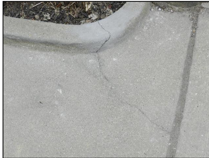
36. Cracked or damaged surfaces
