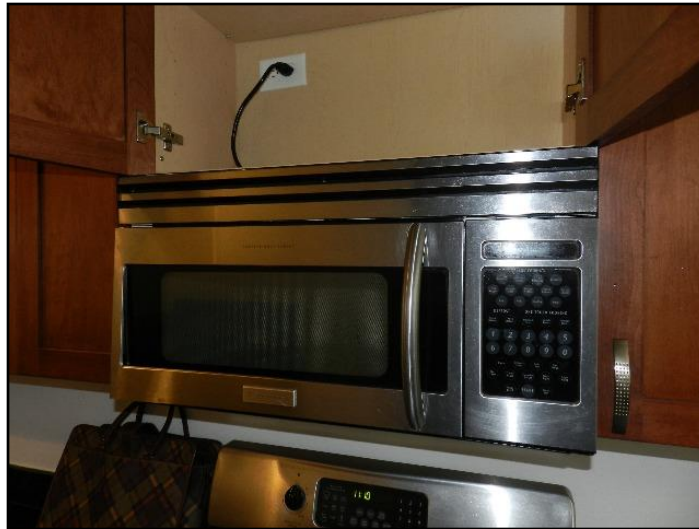
109. Not vented to exterior
