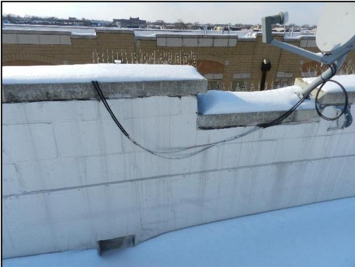
9. Inspect during annual tune-up
