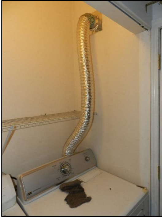
112. Dryer vent material not smooth wall
