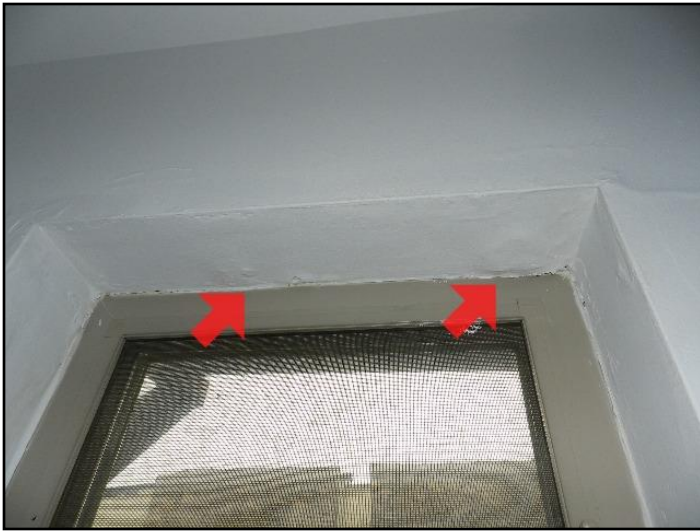
95. Leak at window opening
