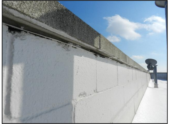
12. Inspect during annual tune-up
