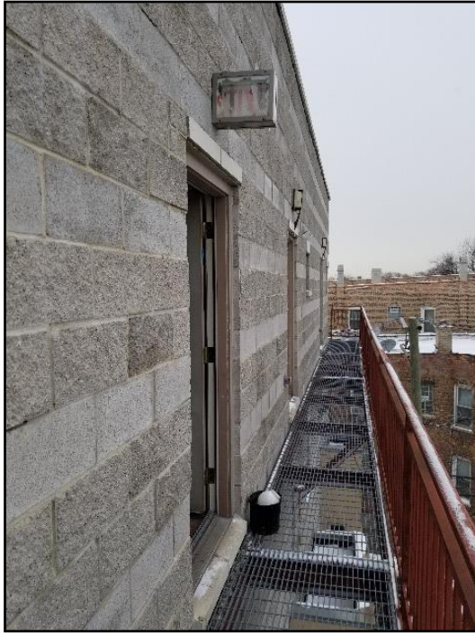
34. Rust at fire escape guard
