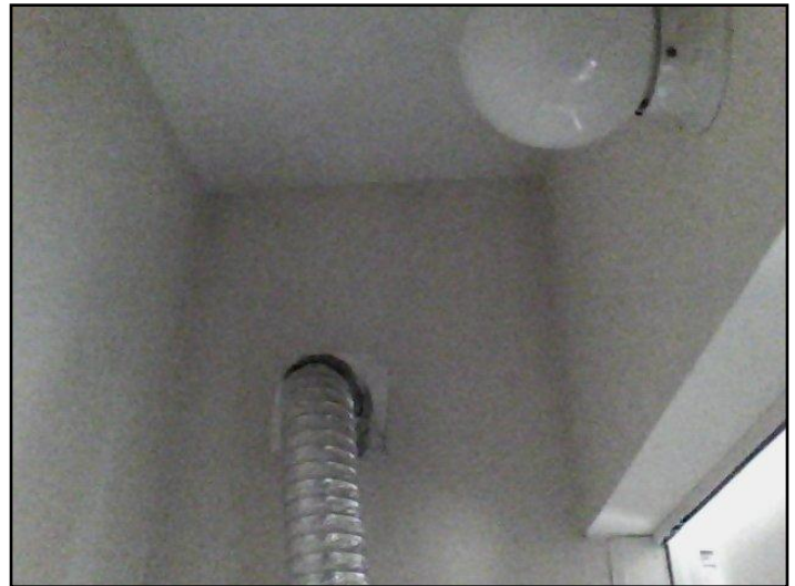
5. Moisture in wall, possible leak
