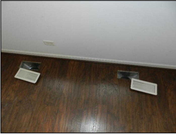
76. Loose, not attached registers
