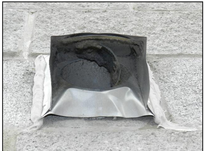
115. Dryer vent material not smooth wall
