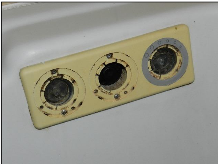
91. Odor, covers missing
