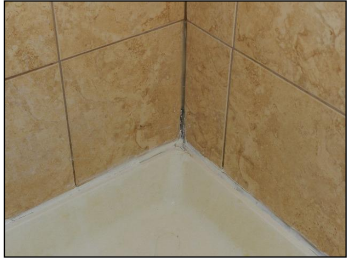
87. Grout loose, missing or deteriorated
