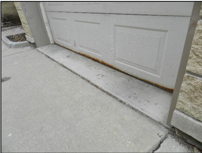
50. Rust, damage to frame
