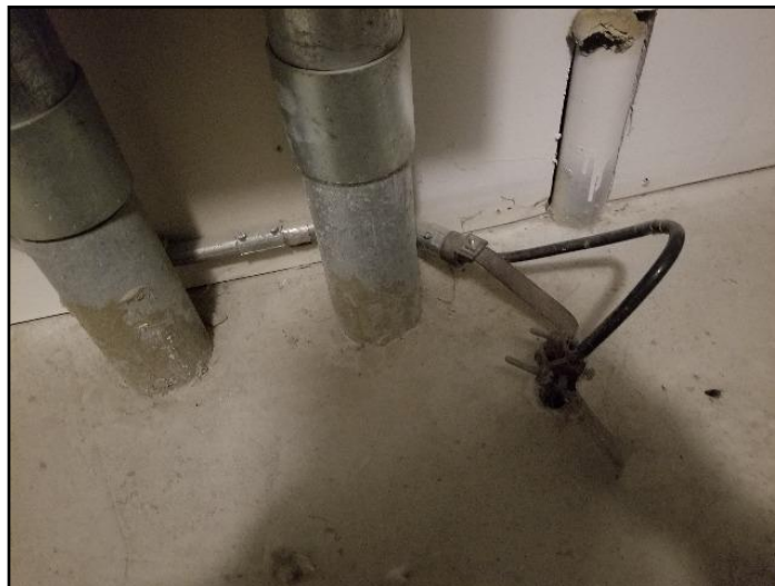
58. Copper - ground rods
