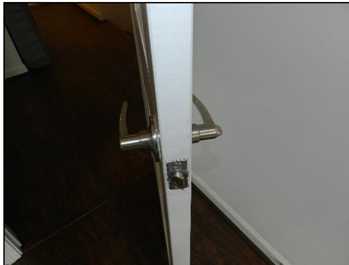
105. Privacy lock broken
