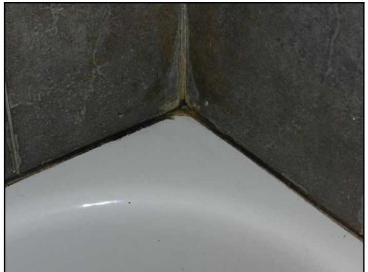
89. Grout loose, missing or deteriorated
