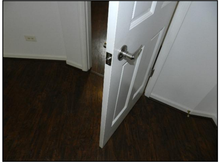
104. Privacy lock broken
