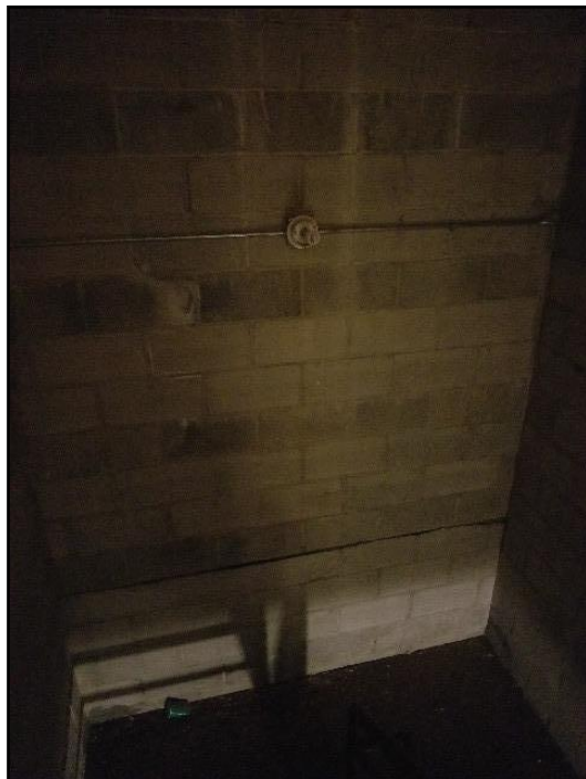
63. Damage, no light at stair
