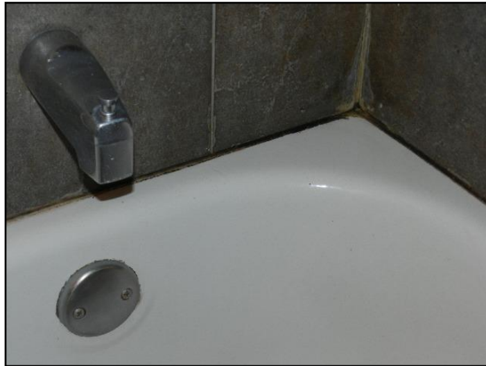
90. Grout loose, missing or deteriorated
