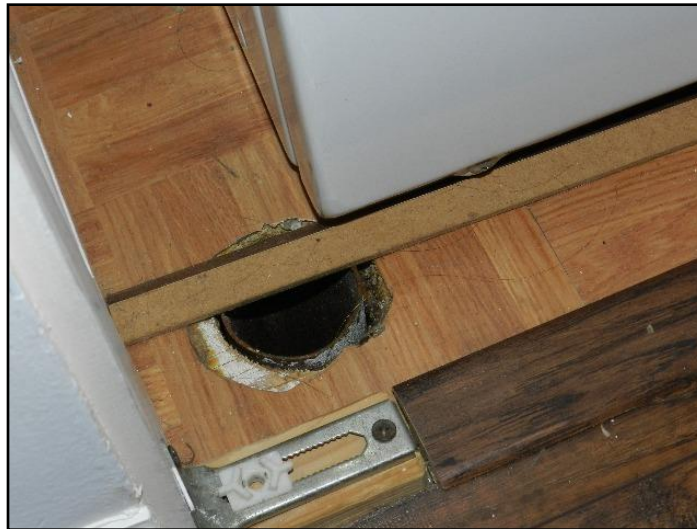
81. Grate missing, rusted or obstructed
