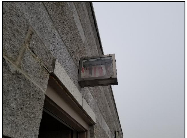
64. Damage to Exit Light
