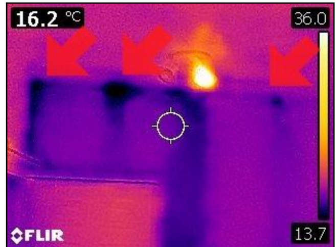
3. Moisture in wall, possible leak
