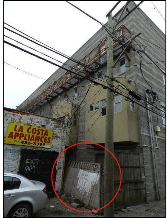
40. Fence damage throughout property
