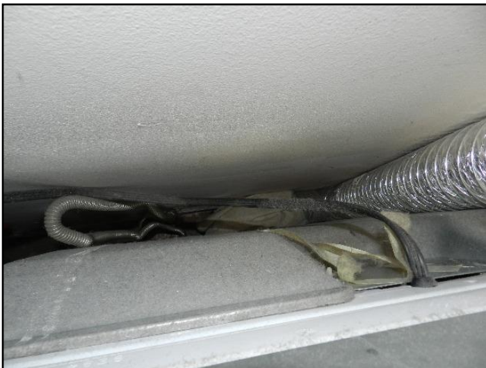
114. Dryer vent material not smooth wall
