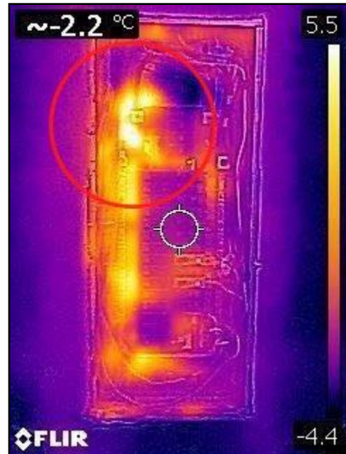
60. Overheating at service feeder
