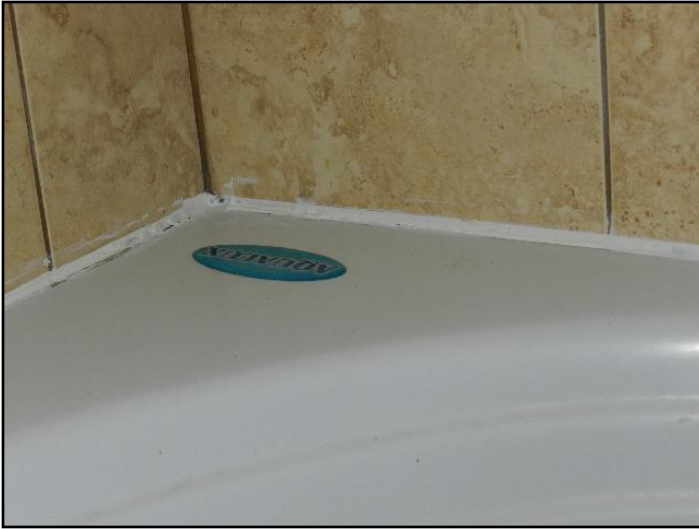
86. Grout loose, missing or deteriorated
