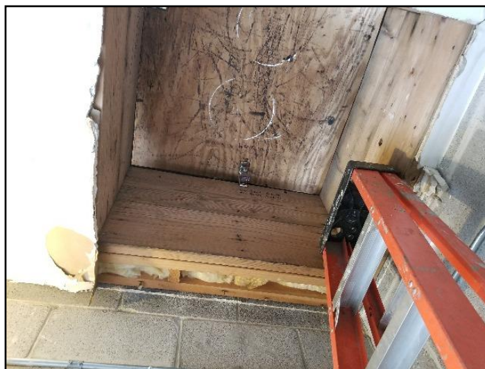
79. Not insulated and not weatherstripped
