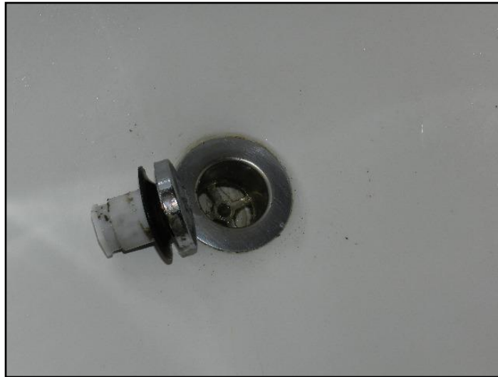
84. Drain stop ineffective
