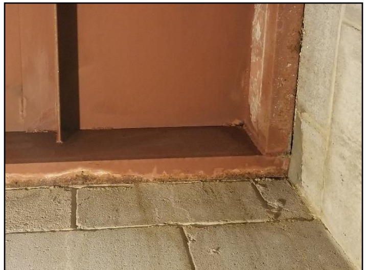
33. Rust at fire escape landing
