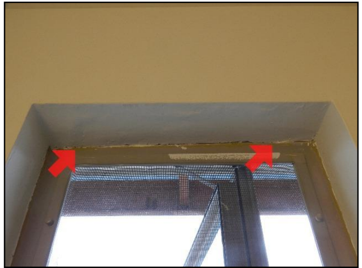
94. Leak at window opening
