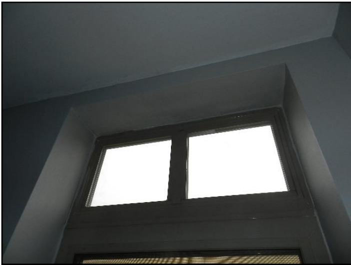
93. Leak at window opening
