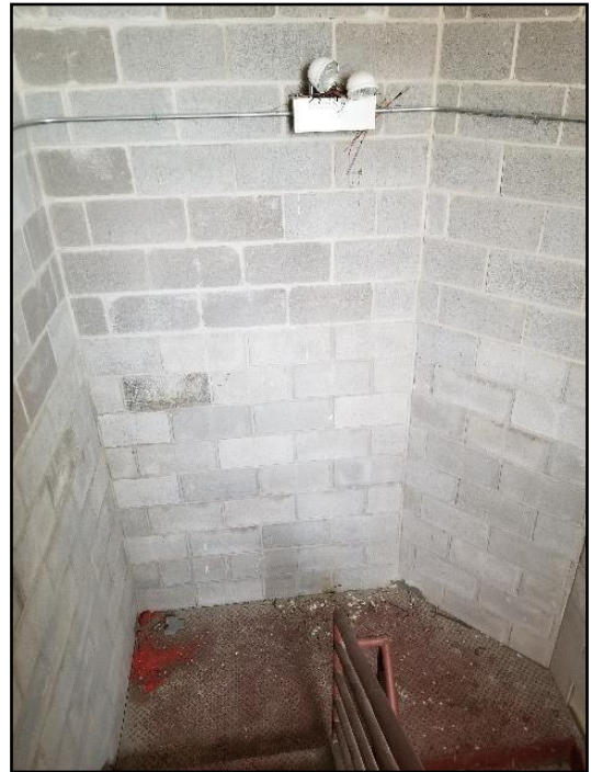
62. Damage to emergency lighting
