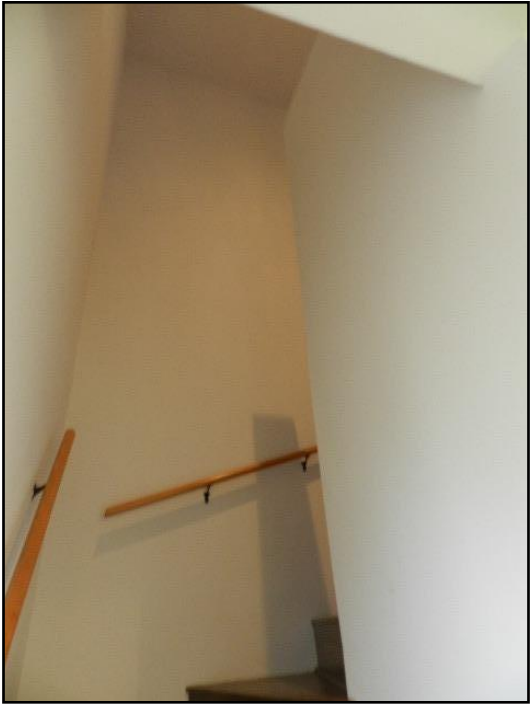
69. Poor stairway lighting
