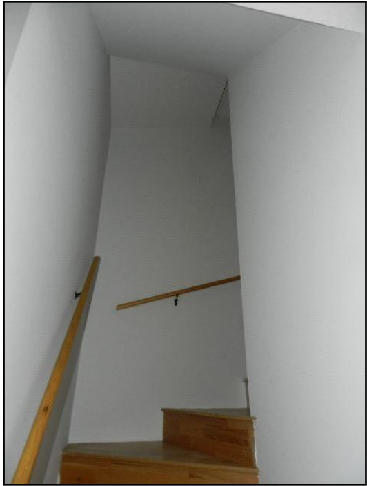
68. Poor stairway lighting
