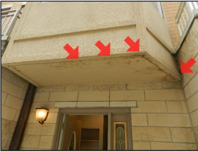
15. No drip edge, water damage
