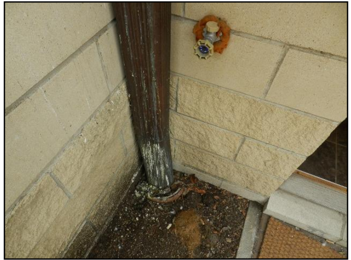
16. Loose or damaged
