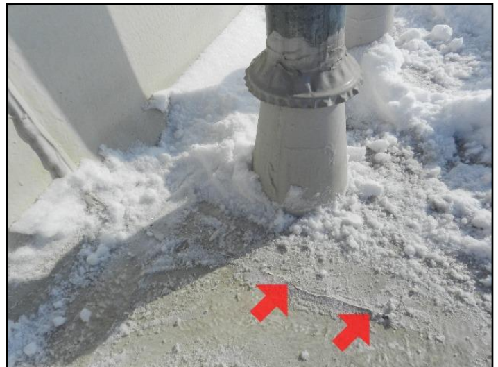
7. Openings at seams or flashings
