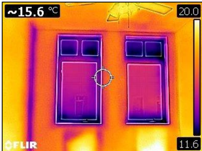
99. Possible water leaks
