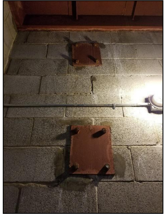
35. Rust at structural support of ledge
