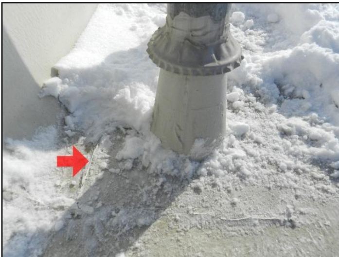
6. Openings at seams or flashings
