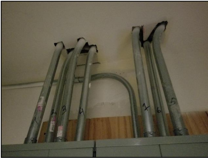
61. No fire caulking/sealant
